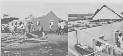
THIS ROOFLESS house was a victim of the tornado. E CAS sin dak aki tabata victima di e hoos cu a pasa like wind that swooped through Pavilla Nov. 6. A similar freak wind cut through Tanki Leendert Nov. 7.
